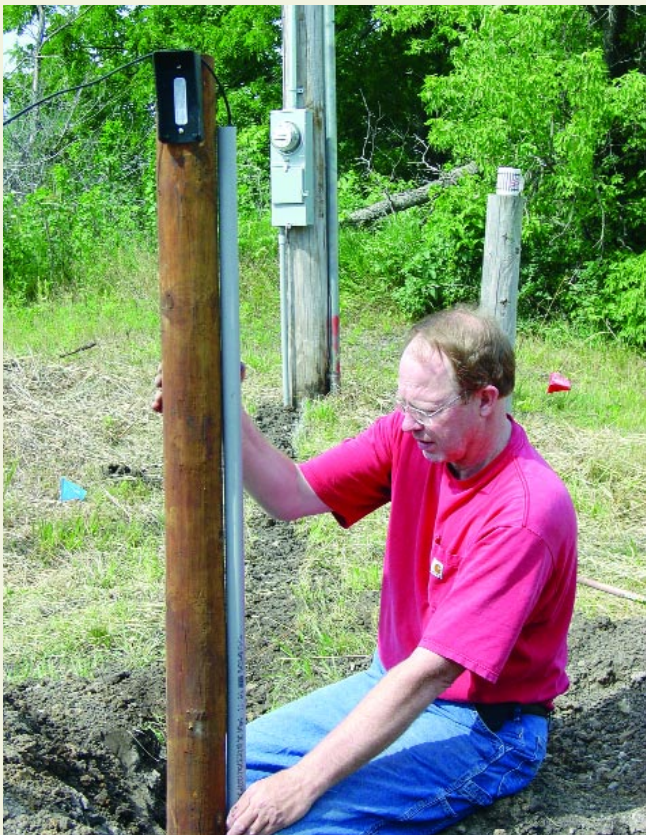
9. Install a key pad post, wiring, and PVC conduit from the key pad to the control box. Note the power supply service and freshly backfilled trench that also leads to the control box. Both lines are in separate conduits.
