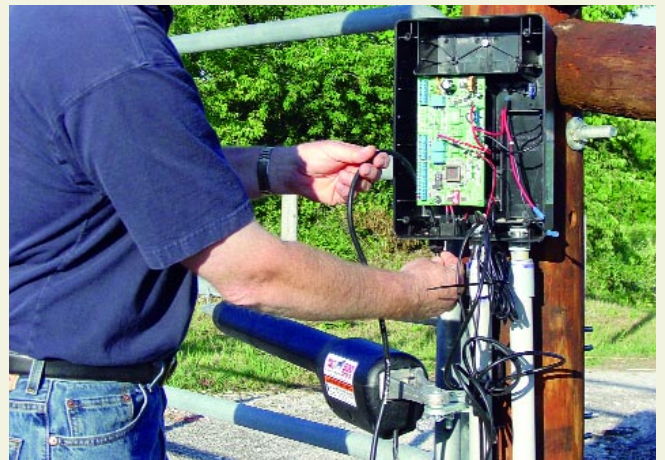
10. An electric control box mounted near the gate hinge post is the brains to the system. All wires run to this box. It is powered by a battery and the battery is charged by either an electric supply line or solar panel.
