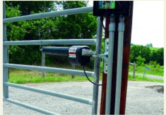
8. Run wiring in PVC conduit from the key pad to the control box, the exit sensor to the control box and the power source to the control box, all in separate conduits. Note the wire running from the control arm feeds directly into the control box.
